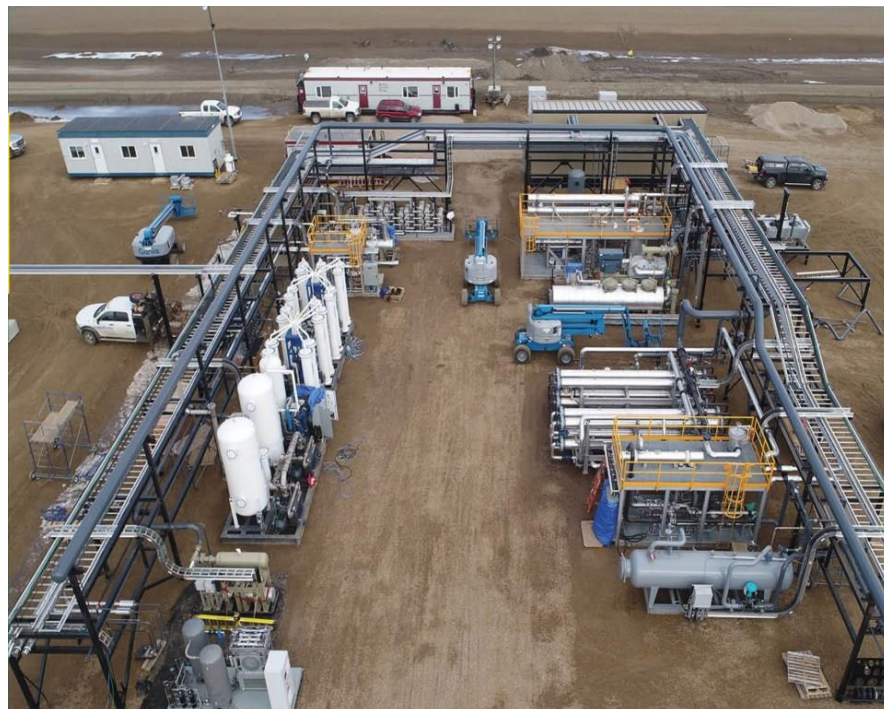
North American Helium Facility, SK Separation Facility (Crude Helium) 20 million standard cubic feet per day
