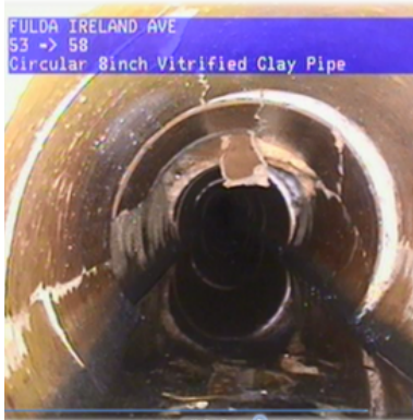
Deteriorated Vitrified Clay Pipe in Fulda, MN
