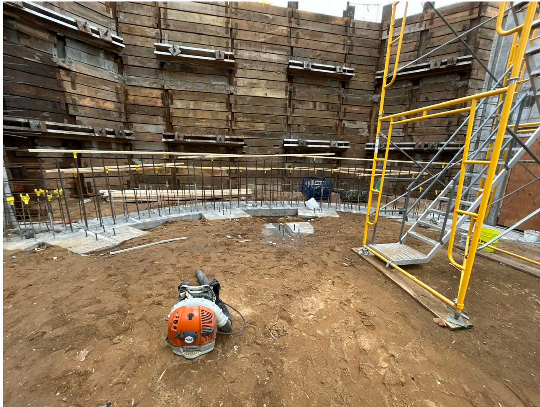
View of concrete footings for arched wall at north end of Zone 1
