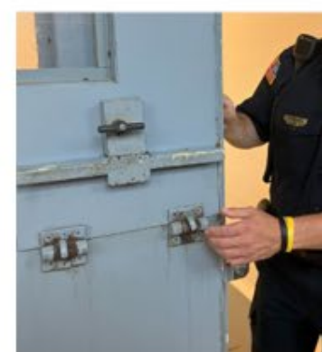
Rusting manual locks on cells
