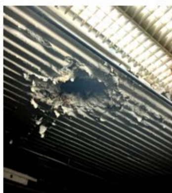
Hole in ceiling that is continuously growing
