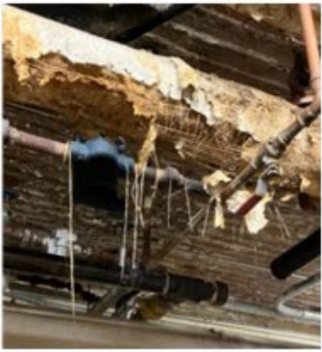
Deteriorating pipes and vents
