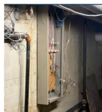
Exposed and outdated electrical wiring
