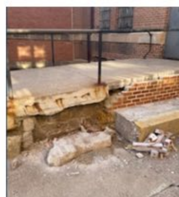
ADA entrance ramp crumbling apart
