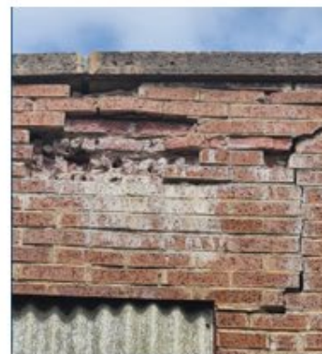
Crumbling brick in outside walls
