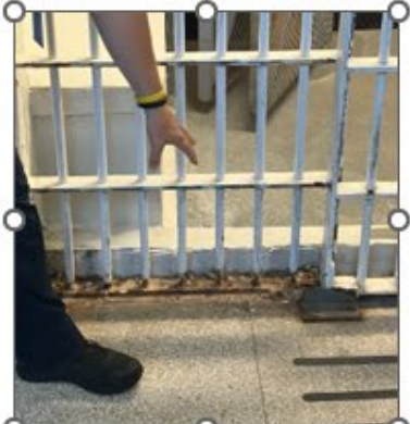
Mold and buildup from cells turned into showers
