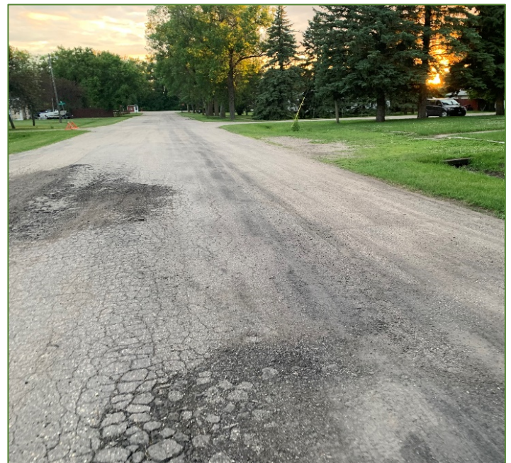
Cracked depressions and loose asphalt on Main Street West in Hendrum
