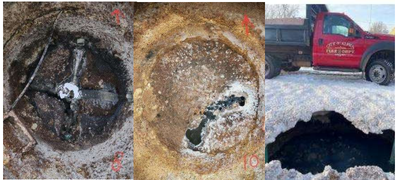
Pictured Above: Damaged and deteriorated manholes.
