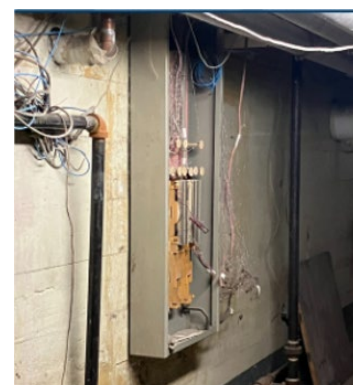
Exposed and outdated electrical wiring
