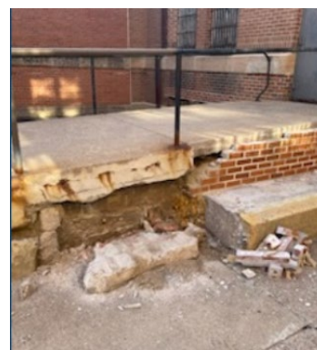
ADA entrance ramp crumbling apart
