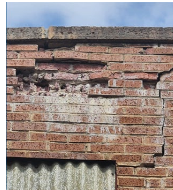
Crumbling brick in outside walls
