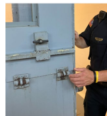
Rusting manual locks on cells
